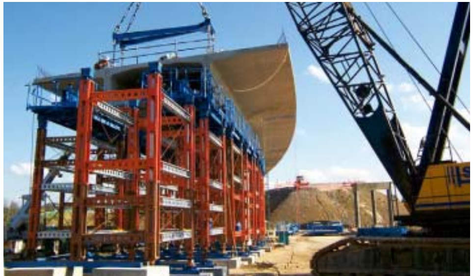
Installation of a bridge segment at the Westlink M7 motorway interchange for the M5 motorway.
