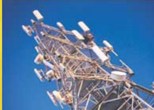
Vodafone base stations Homebush Bay, New South Wales
