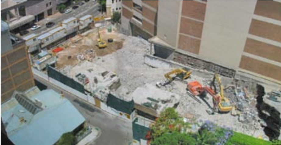
Excavation of the footprint for 100 Pacific Highway is now well advanced with the last vestiges of the previous structure being removed and the car park excavation due to start
