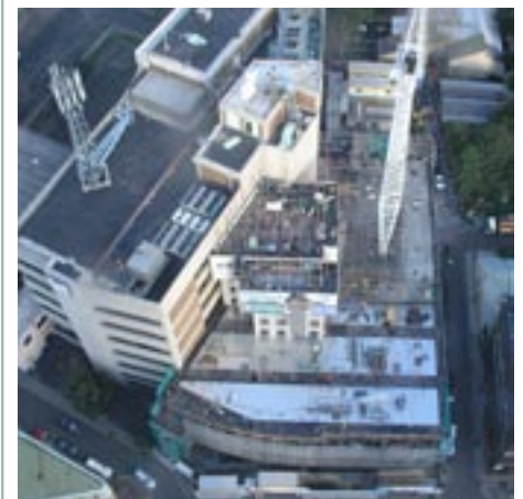
The development is now taking shape and will create a striking addition to the North Sydney skyline
