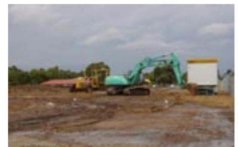
Preliminary works begin on site at the Peninsula Homemaker Centre, Mornington with the removal of excess spoil and bulk earthworks to the building pads
