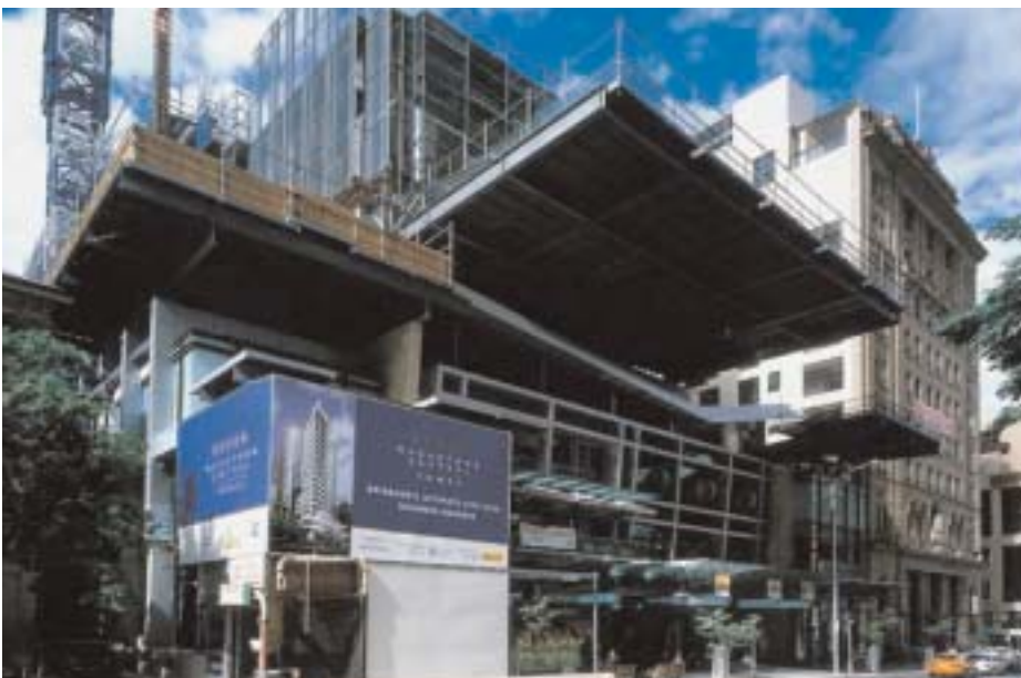
The MacArthur Central Retail Complex will prove to be a landmark development and one of Brisbane's best locations to work and shop
