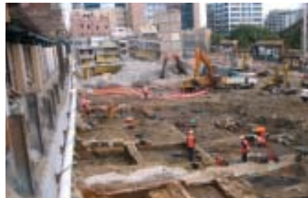
Foundations of the 'Sydney & Melbourne Hotel', with associated buildings (cnr of Kent and Napoleon Streets)
