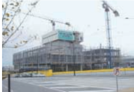
Work on 700 Collins Street is progressing well and is on schedule for completion by mid-2004
