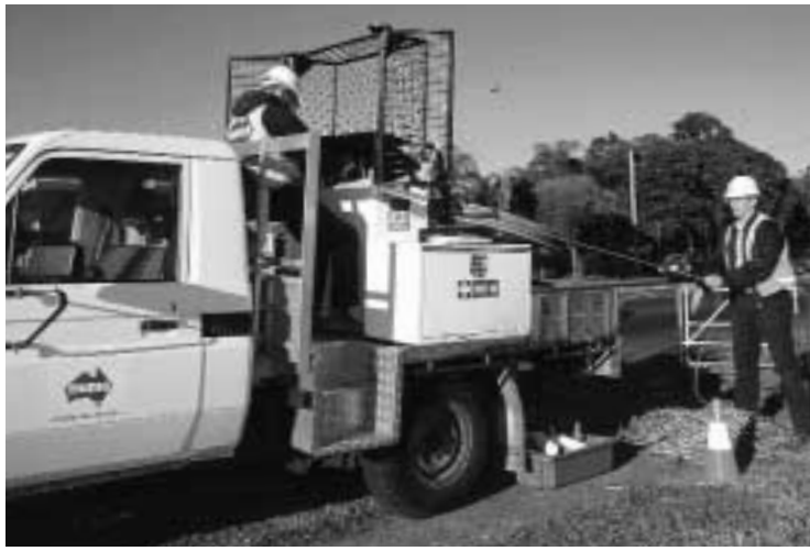
Telstra's Customer Access Network Access Renewal, New South Wales and Queensland, Thiess
